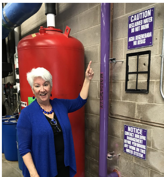
Travis County Commissioner and Clean Water Action board member Brigid Shea points to the downtown library's alternative water setup. The library uses AC condensate and rainwater for irrigation, toilet flushing and cooling tower make-up water, as will the new Travis County Courthouse.
